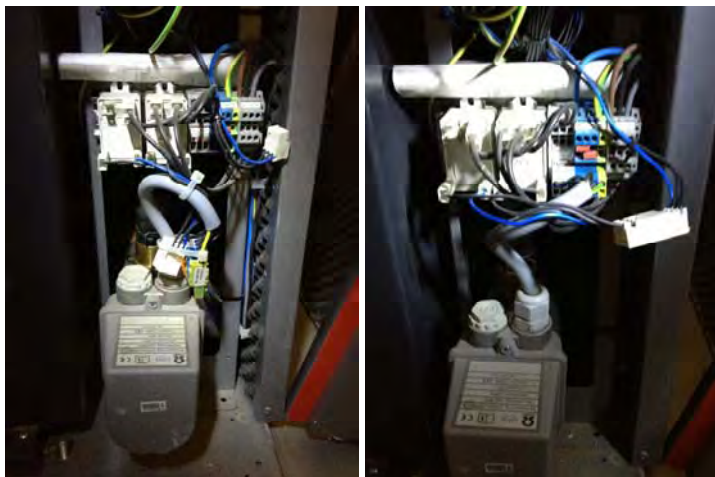
Figure 3-12 The GSHP direct heater as found in May 2013 (left), and after it was connected (right)
