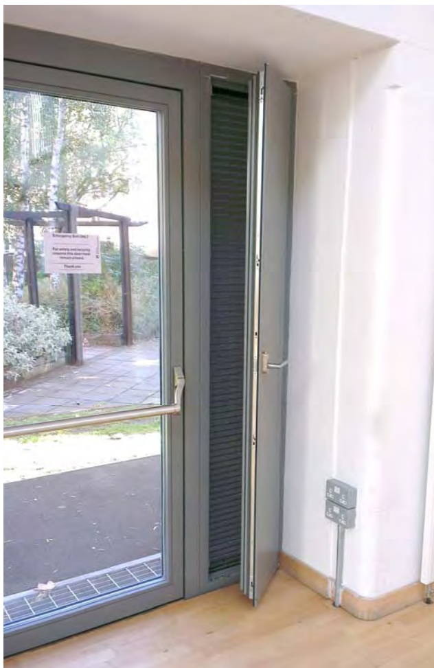
Figure 5-5 Ventilation grille (main hall)
