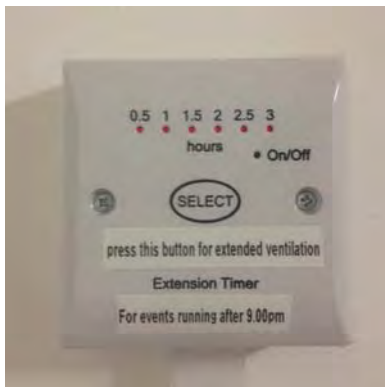
Figure 3-6 Ventilation extension timer (basement, main staircase hall)
