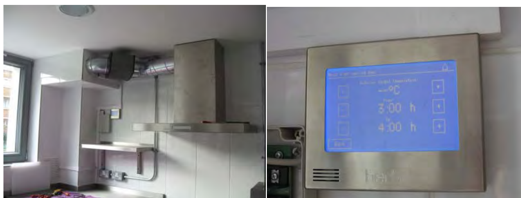
Figure 3-7 Kitchen hood, filter and controls display
