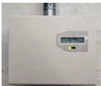
Figure 3-4 CO 2 sensor (main hall)
