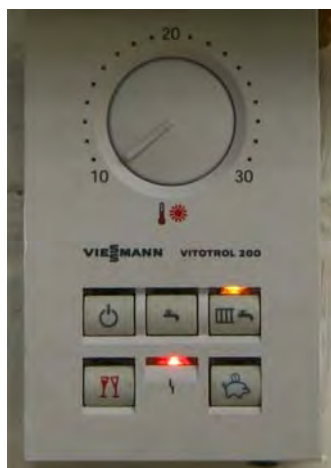
Figure 3-10 Thermostat and DHW & heating controls (main hall)
