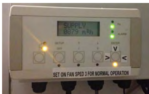
Figure 3-2 Ventilation unit – controls display (plant room)
