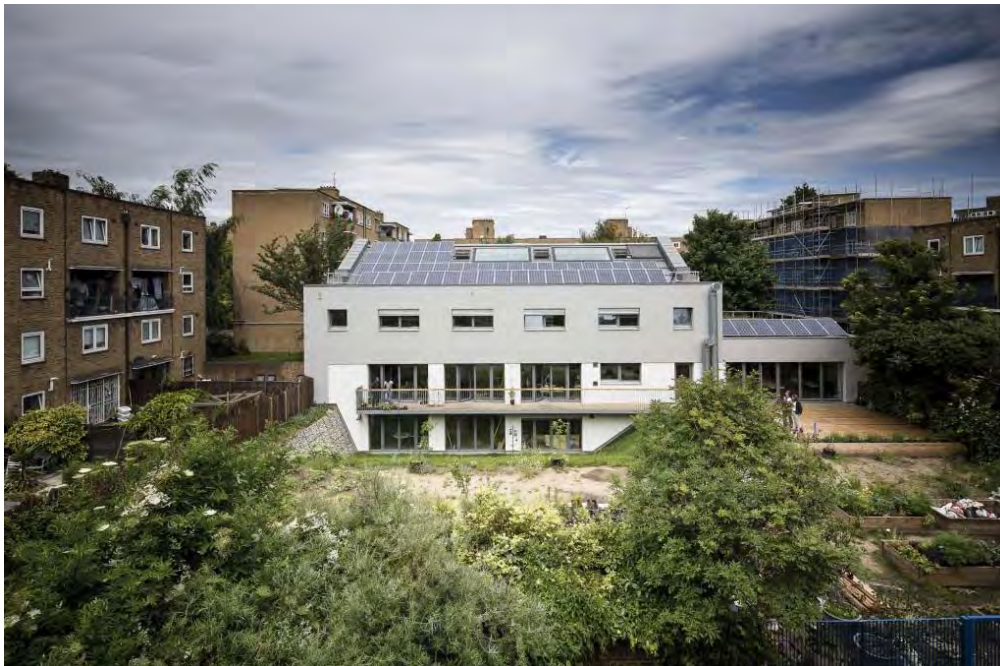
Figure 3-14 Mildmay Centre - photovoltaics arrays (on the main zinc roof and on the ground floor extension)
