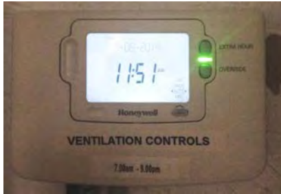
Figure 3-5 Ventilation timer control unit (plant room)
