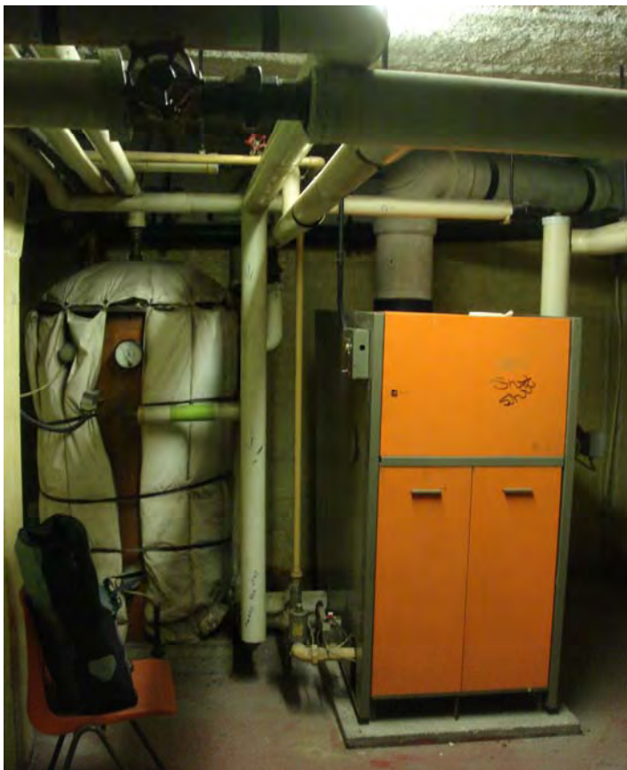
Figure 2-3 Gas boiler and tank in the basement of the Centre prior to refurbishment
