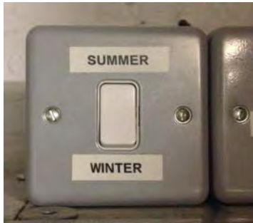
Figure 3-3 Ventilation unit – summer/winter strategy switch (plant room)
