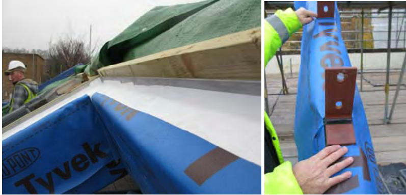
Figure 2-13 Airtightness tapes around windows (previous page) and thinking ahead with membranes fitted to rooflights and trusses in readiness for later connection to the main membranes.
