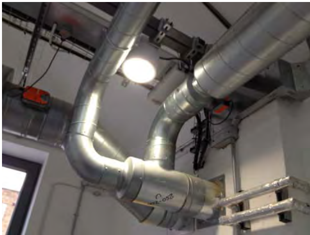
Figure 5-7 First floor ventilation ductwork
