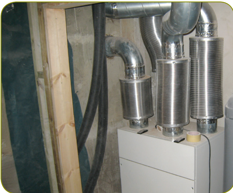
Figure 3.4: MVHR unit showing input and exhaust ducting with silencers
